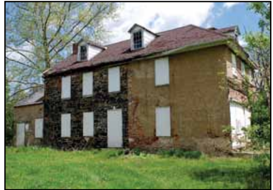
Evans House, 2010, with the roof noticeably in need of repair.
